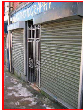
This is a bad example of a solid metal roller shutter with external housing box in galvanised metal finish
