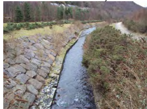
Plate 4 Ebbw Fach River at culvert outlet, to the south of the site, looking downstream (south)
