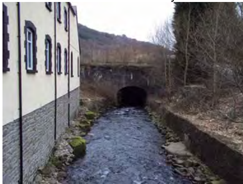
Plate 3 Ebbw Fach River and culvert, looking downstream (south). The building on the left is the Six Bells Baptist Church
